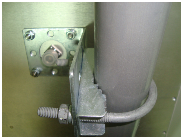
Mount Secured to Pole/Mast
